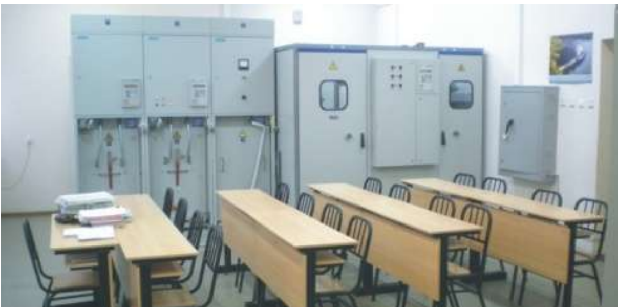
Pic. 5. Block traction substation laboratory overview
